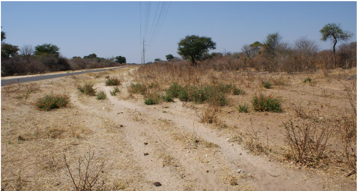
Figure 5: Baikiaea plurijuga – Pterocarpus angolensis bushlands after being cleared, under the powerline towards Katima Mulilo (plot C5). Note the relative low regrowth of shrubs.
