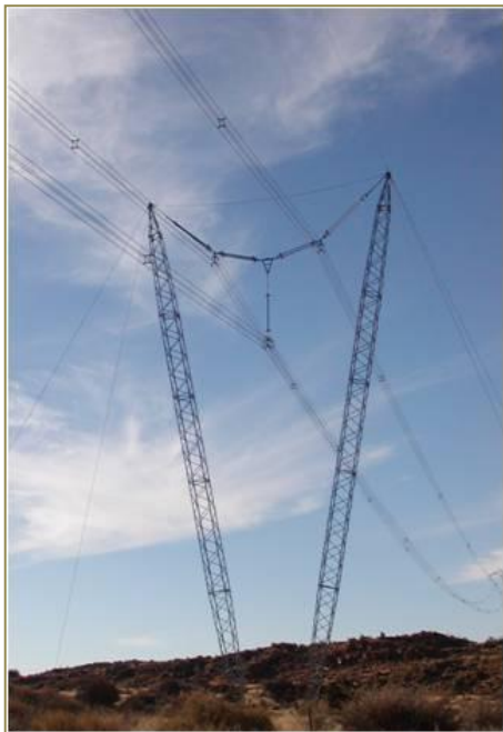
Figure 2: An example of the proposed structures to be used for this transmission line.
