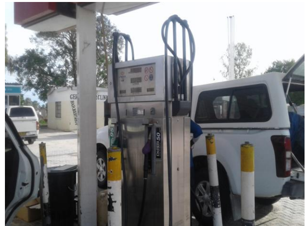
Photo 4. Double-hose pump (ULP and 50ppm Diesel)
