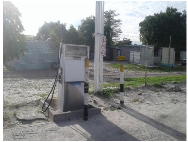
Photo 2. Existing COC pump and vents
