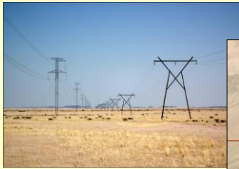
Parallel line structures on the Trekkopje Bypass: 220 kV steel pylon (left/south) and 66 kV wooden pole Kamerad (right/north).
