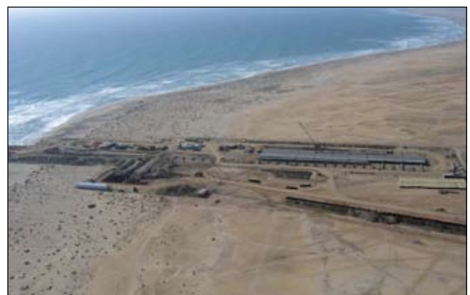
Below: Construction of the first desalination plant for the uranium mine of Trekkopje in the Erongo region (© N. Cadot)
