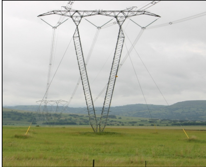
Figure 2: Guyed-V Suspension Tower
