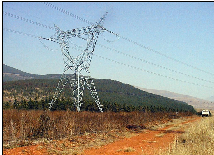
Figure 3: Self-Supporting Strain Tower
