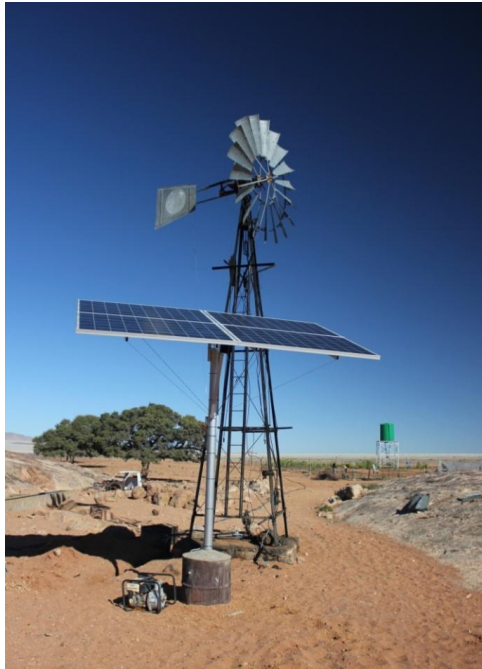
The new solar powered water pump
