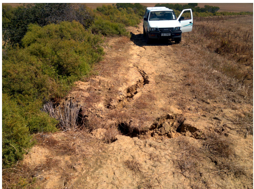
Figure 4: Bank gully expansion along farm dirt road
