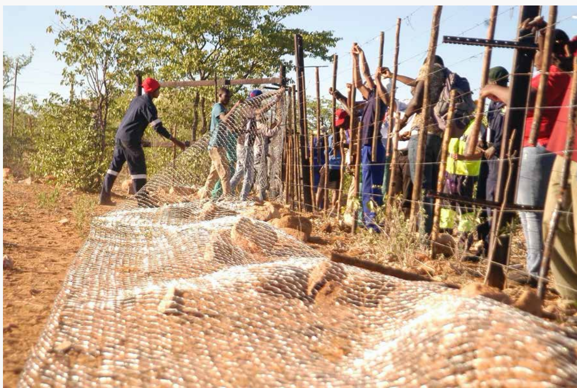
Youth volunteers constructing sections of the Etosha National Park Fence during the 12th National Youth Week.
