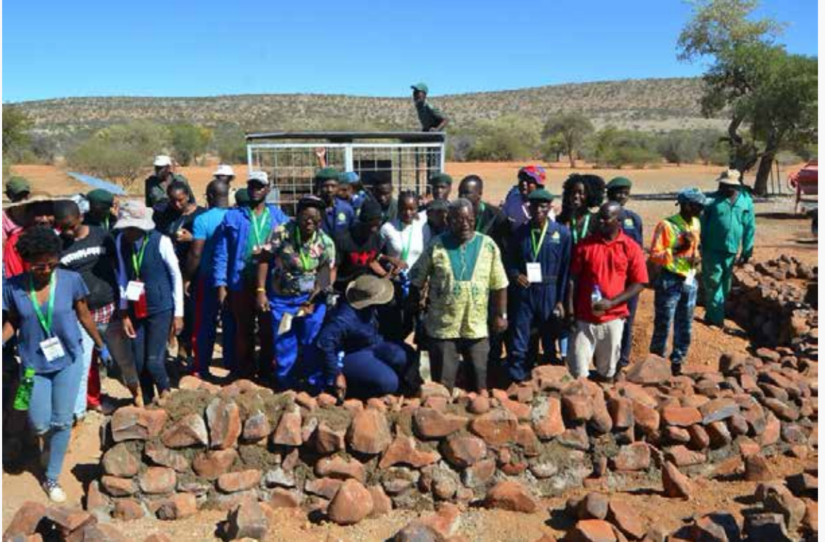
Youth volunteers constructing elephant protection walls for local conservancies during the 12th National Youth Week.
