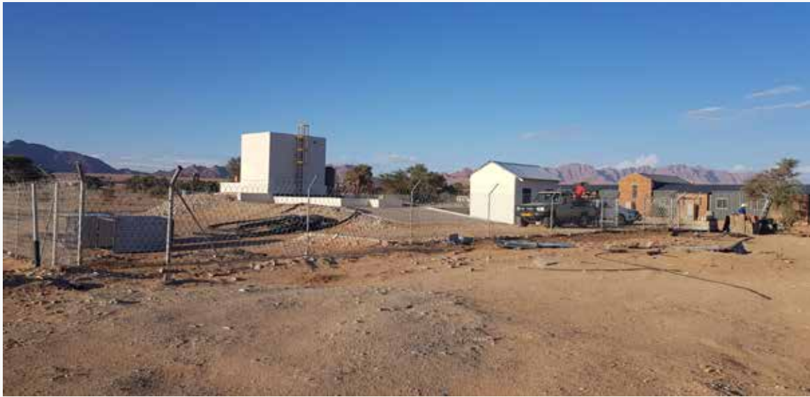
Upgraded sewerage facility and water supply system at Sesriem in the Namib Naukluft Park.
