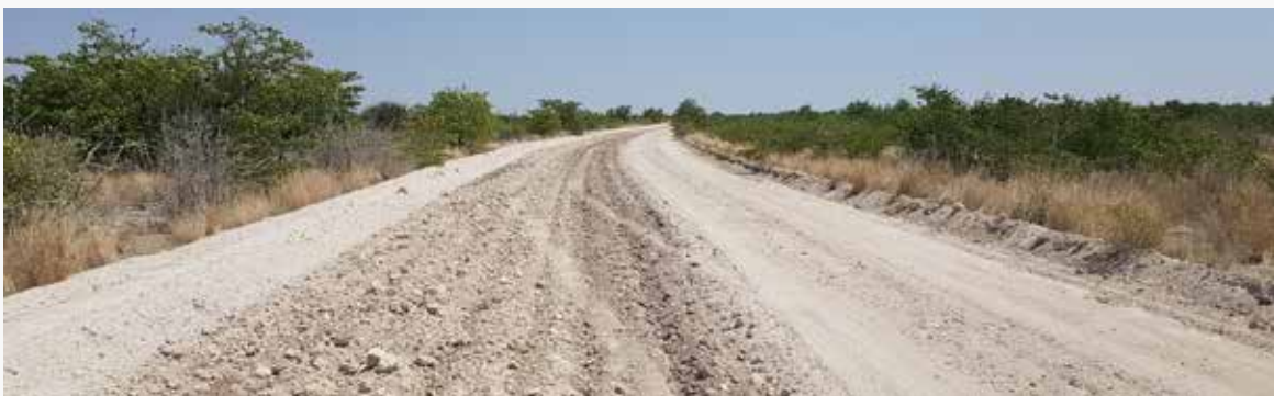
Rehabilitation work being undertaken on the Okaukuejo - Otjovazandu road in Etosha National Park.
