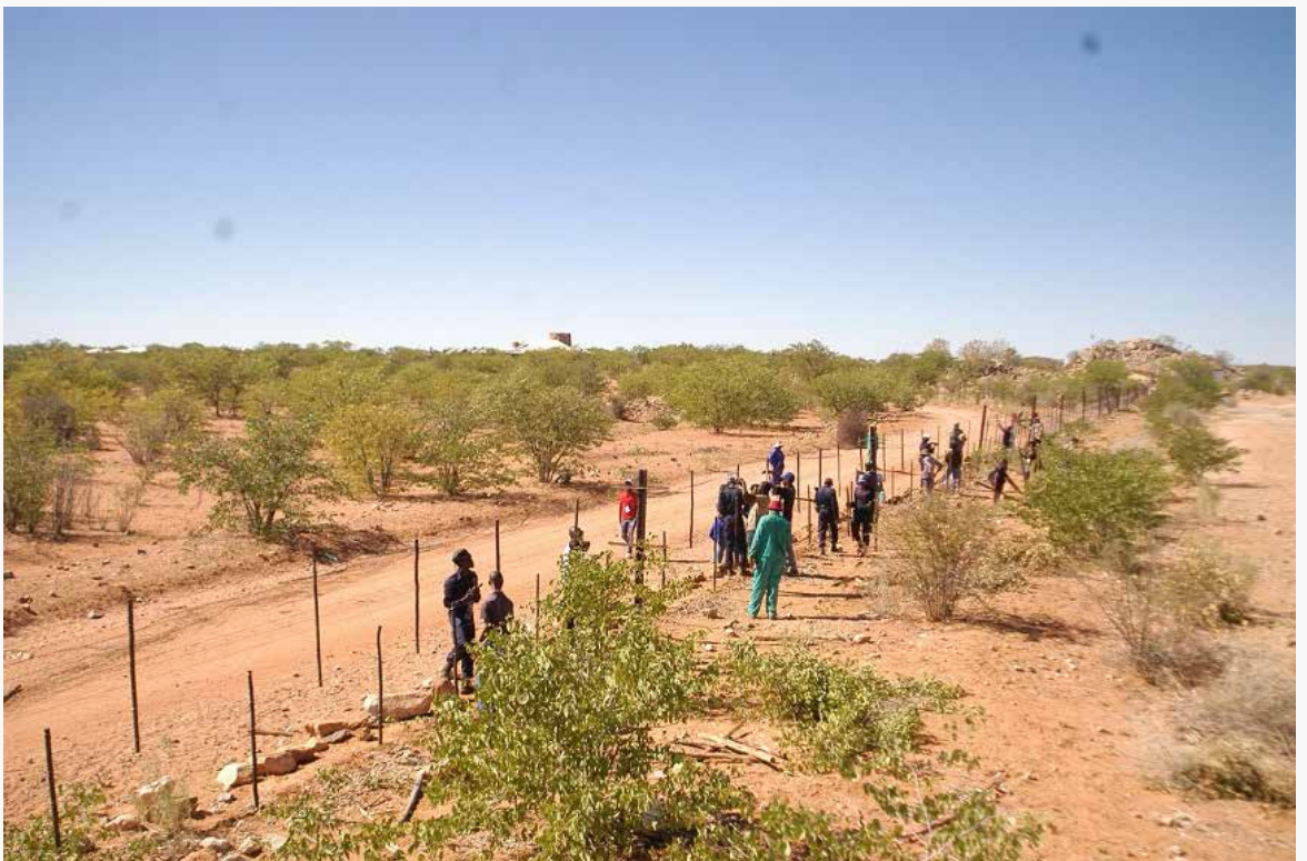
Repair work on the Etosha National Park fence during the 12th National Youth Week.
