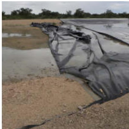
(a) Damage to the oxidation pond lining increases the risk of groundwater contamination
