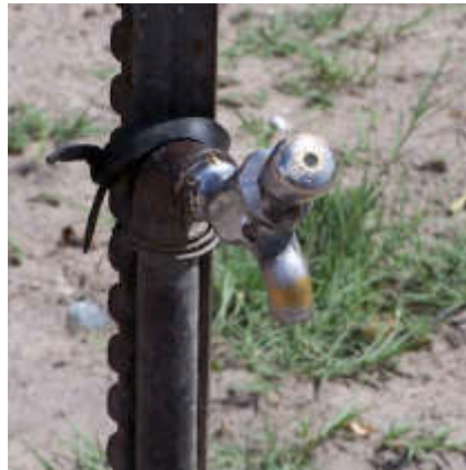
Figure 2.4: This self-closing tap opens only when the button is depressed, preventing it from being left open and forgotten
