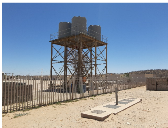
Photo 12. Water storage and oil/water separator
