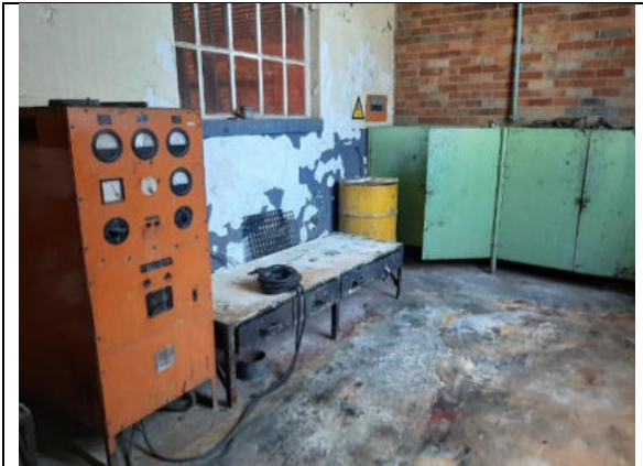
Photo 4-7 Battery charging station
