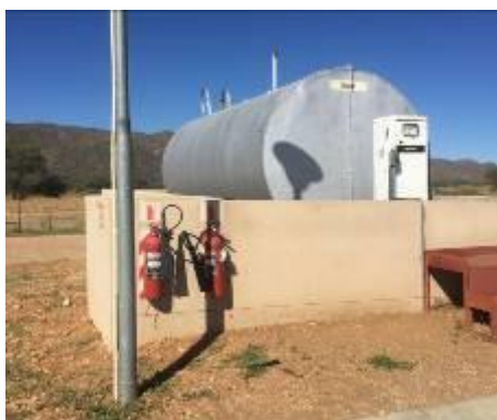
Figure 5: Diesel storage container
