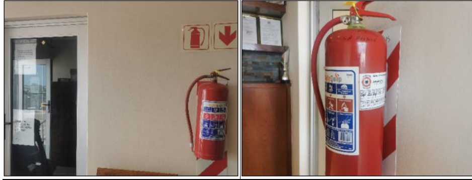
Figure 2-9: One of the many fire extinguishers onsite
