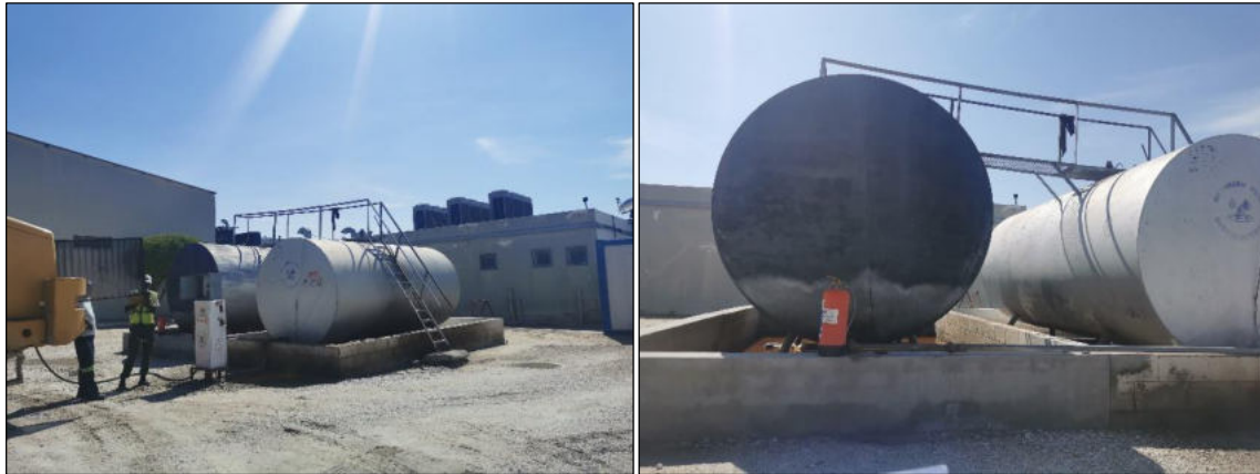
Figure 2-6: The two 23,000-litre diesel tanks onsite
