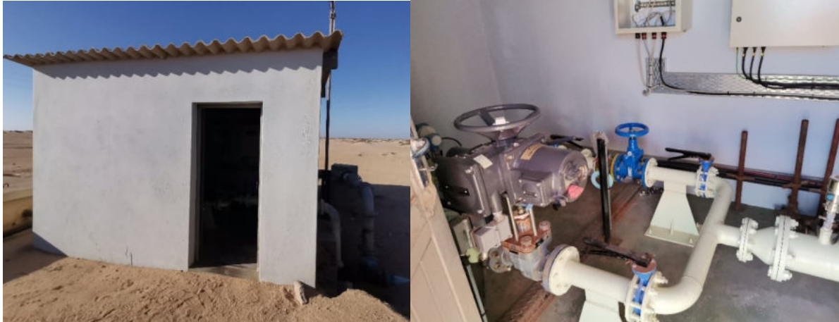
Figure 5: Facilities at the Off- take
