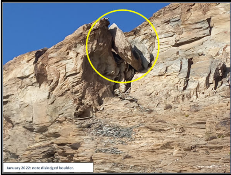
Figure 5: Rock showers – Dislodged boulder.
