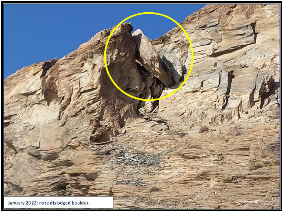
Figure 5: Rock showers – Dislodged boulder.
