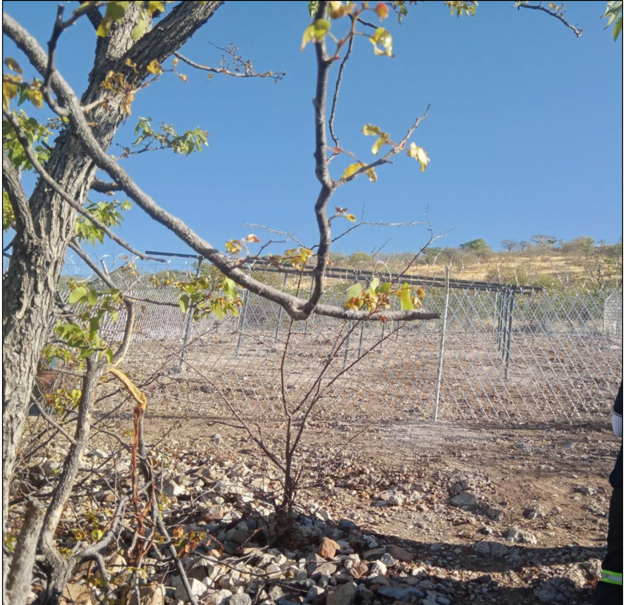
Figure 5: Shows the fenced off stands where 28 solar panels will be mounted.
