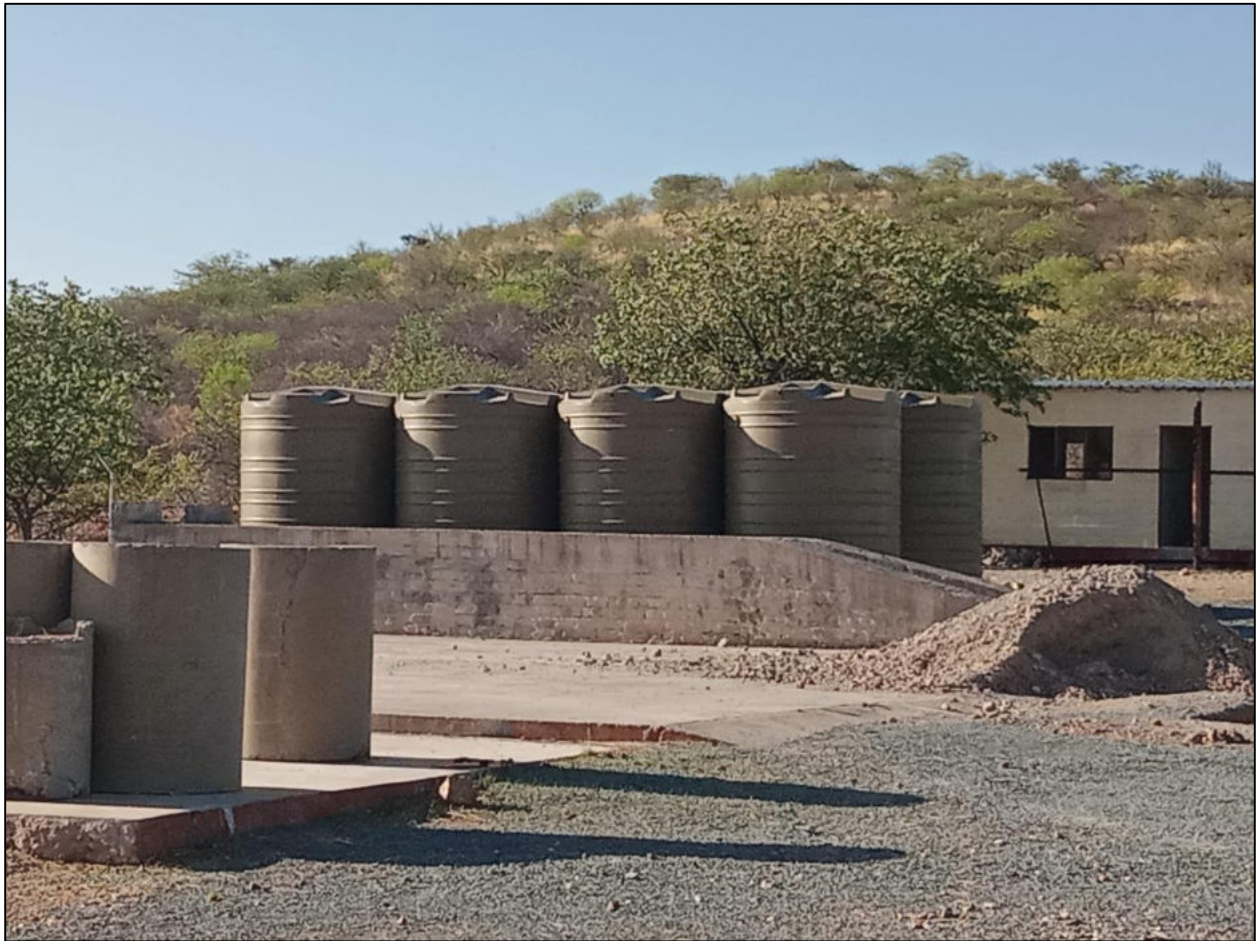
Figure 4: 8x10 000 litres water tanks on site.
