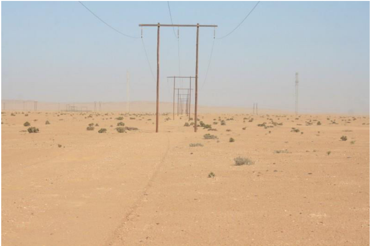
Figure 2: The 66kV Kuiseb-Langer Heinrich transmission line
