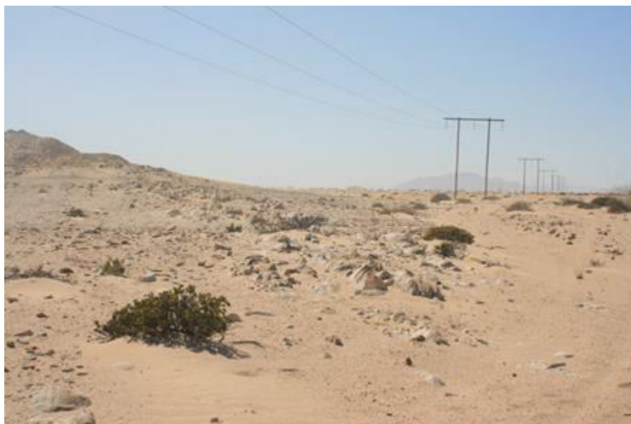
Figure 7. Rocky ridge with white/grey geology encountered under the line along the route is viewed as “medium” sensitivity area.
