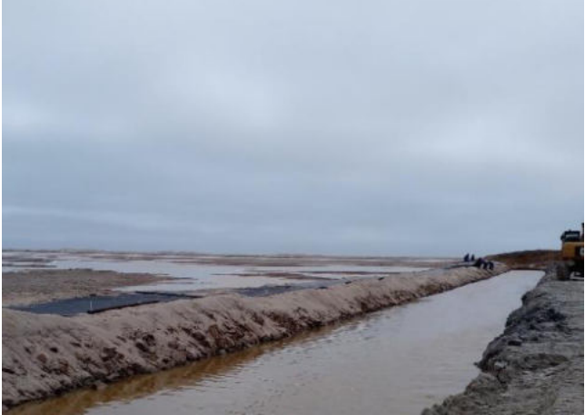
Wash water canal
