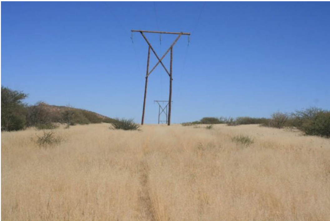
Figure 2. The 66KV Marble-Navachab transmission line.
