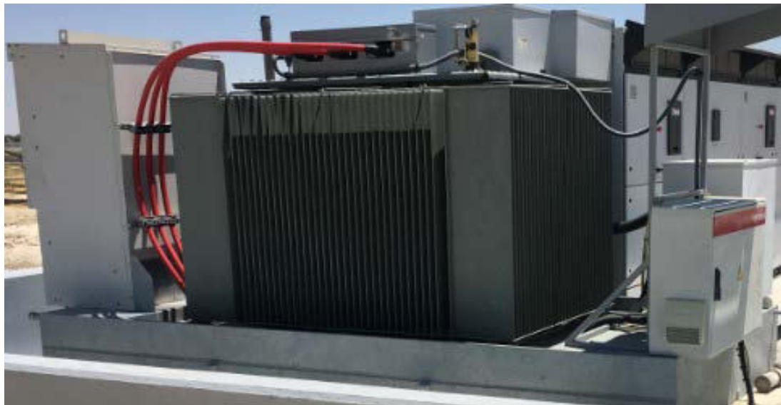
Photo 4.2 – Example of a field transformer
