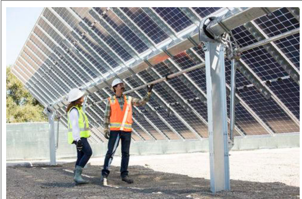
Photo 4.1 – Example of single axis tracking system
