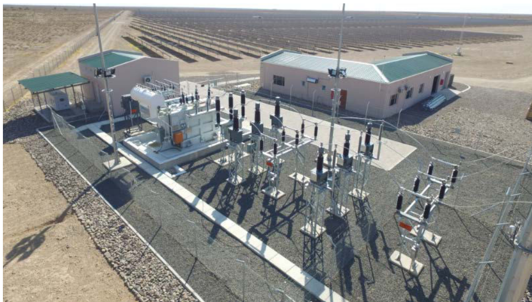
Photo 4.3 – View of a similar site substation & buildings
