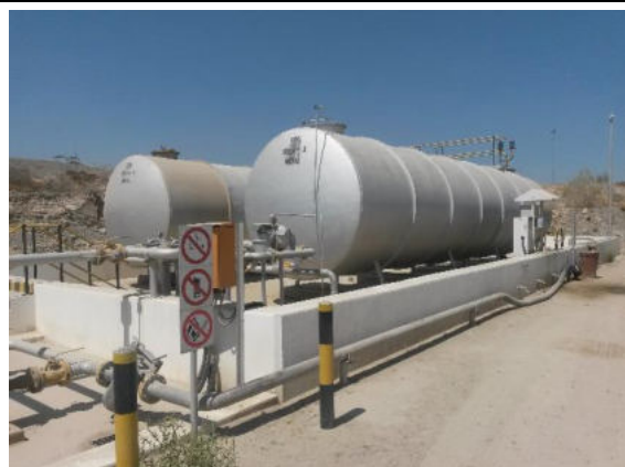
Photo 1 Existing diesel storage tanks
