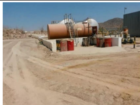
Photo 2 Used oil tank and diesel storage tanks.
