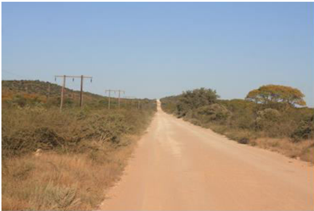
Figure 2. The 66kV Otjikoto – Tschudi transmission line with H – Pole structures
