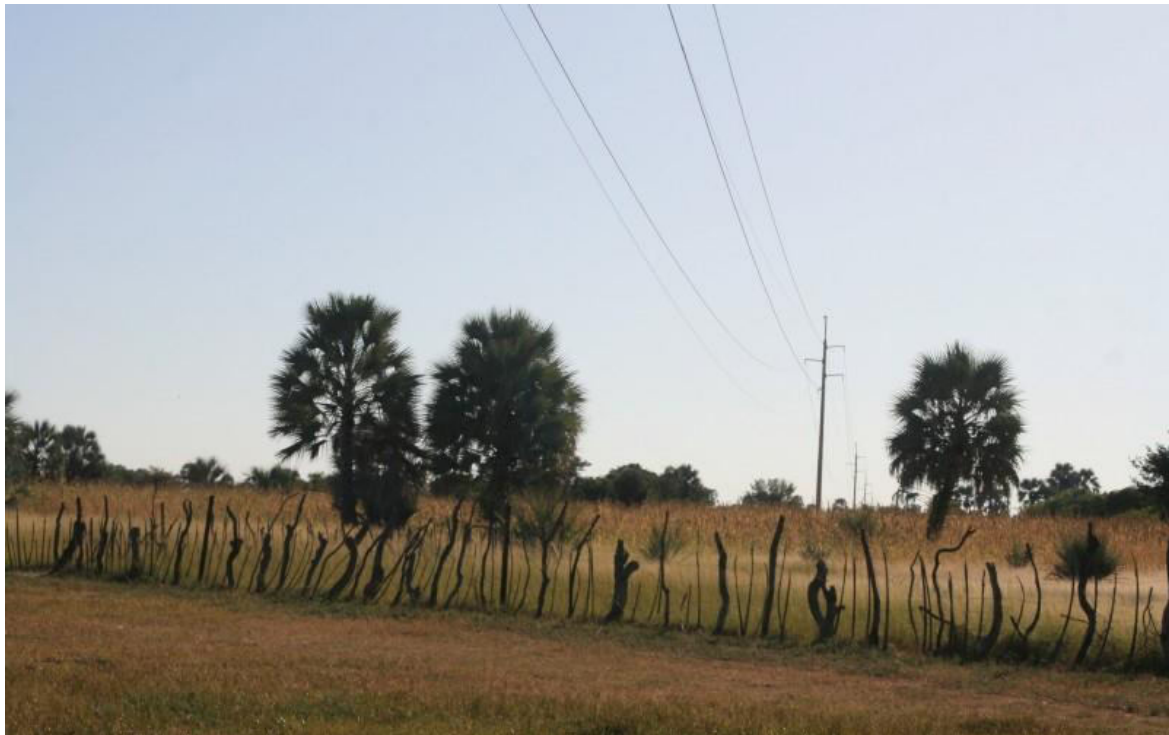
Figure 2: The 132kV Efundja – Ondjiva Transmission line with guyed steel monopole structures traversing through mahangu fields
