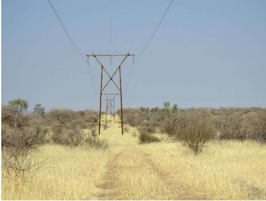
Figure 5 - Proposed overhead powerline will be similar to the example in the figure.
