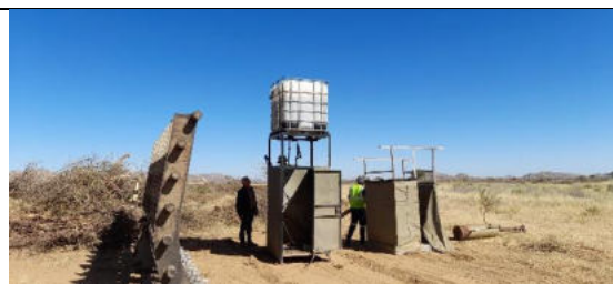
Photo 3-8 Establishment of ablution facilities
