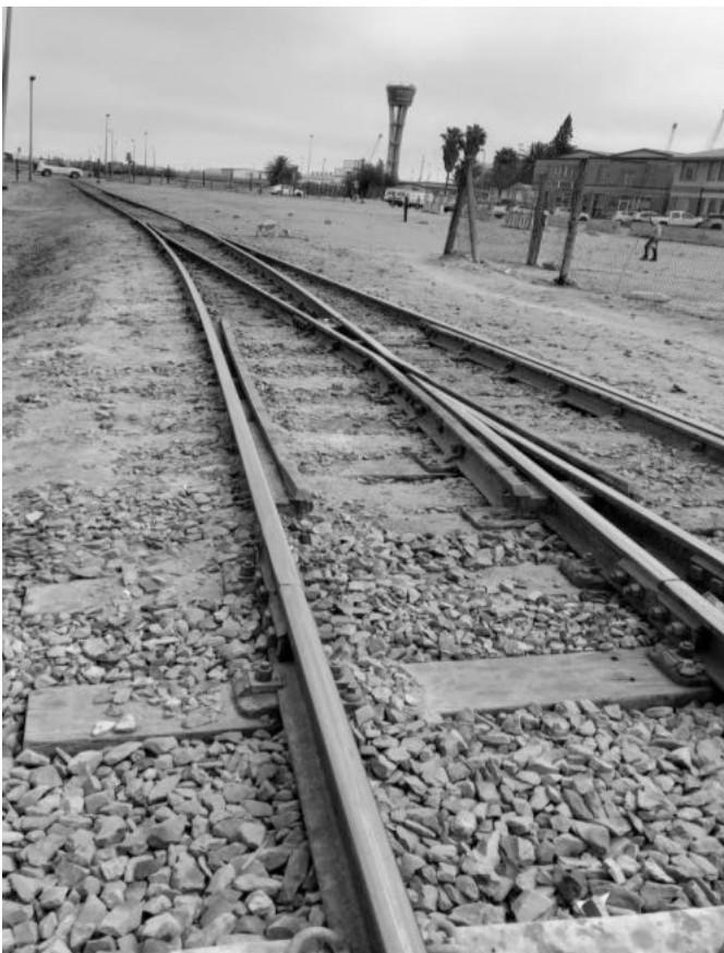
Figure 3 - Condition of the fuel line turnout, leaving NamPort.
