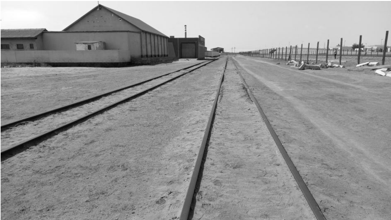
Figure 4 - Condition of the fuel line. On the far right the upgraded railway line.
