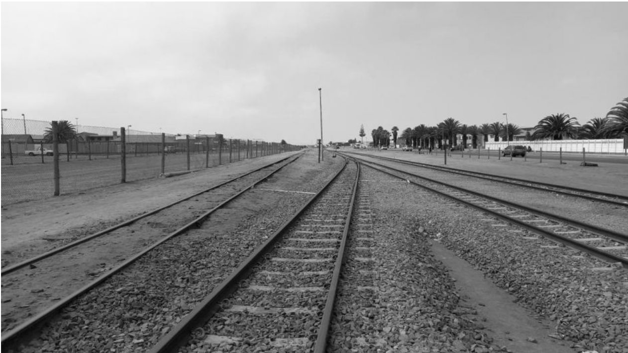
Figure 2 - Condition of the upgraded railway line (middle and right) in comparison to the fuel line (left), leaving NamPort.
