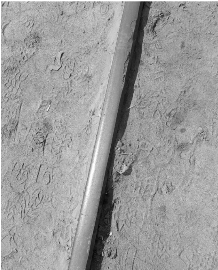
Figure 5 - Safety concerns on the track for the rails of the TransNamib locomotives.
