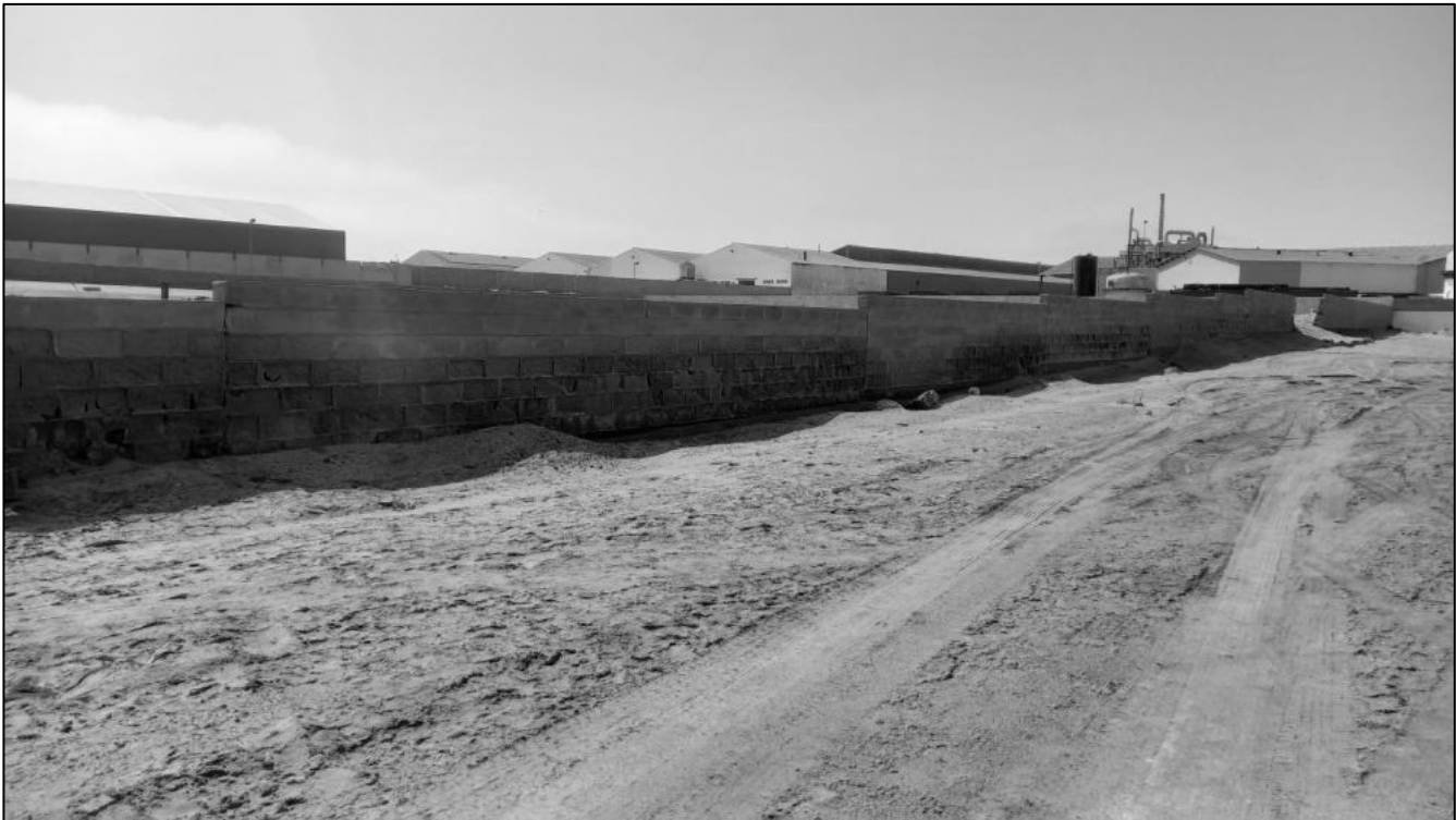
Figure 12 - Visual overview of the current condition of the Old Walvis Bay cemetery (boundary wall).
