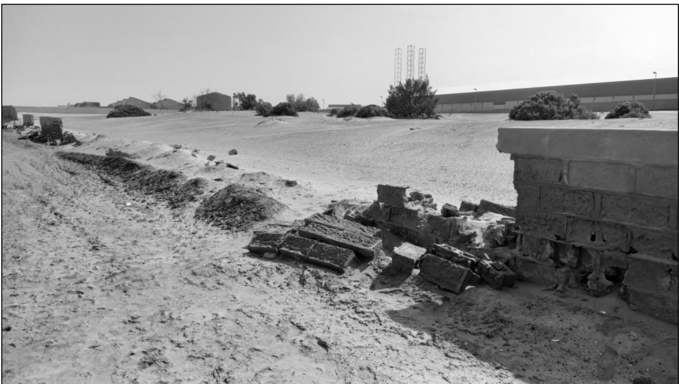
Figure 13 - Visual overview of the current condition of the Old Walvis Bay cemetery (including wall).
