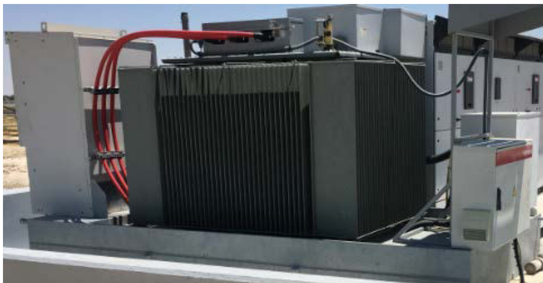
Photo 4.2 – Example of a field transformer
