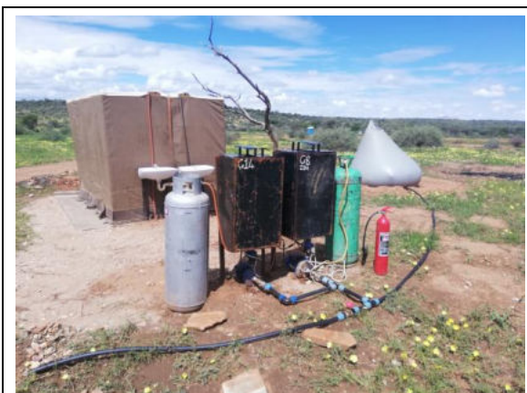
Photo 4-3. Gas geysers and fire extinguisher
