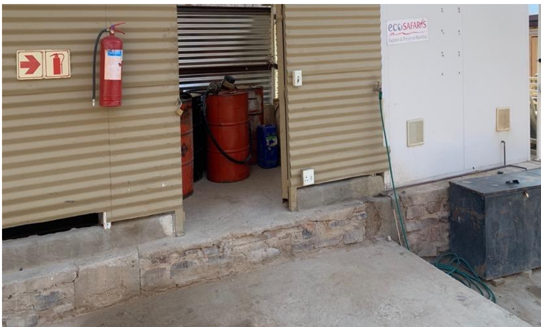
Figure 15. Diesel storage with battery room to the right.
