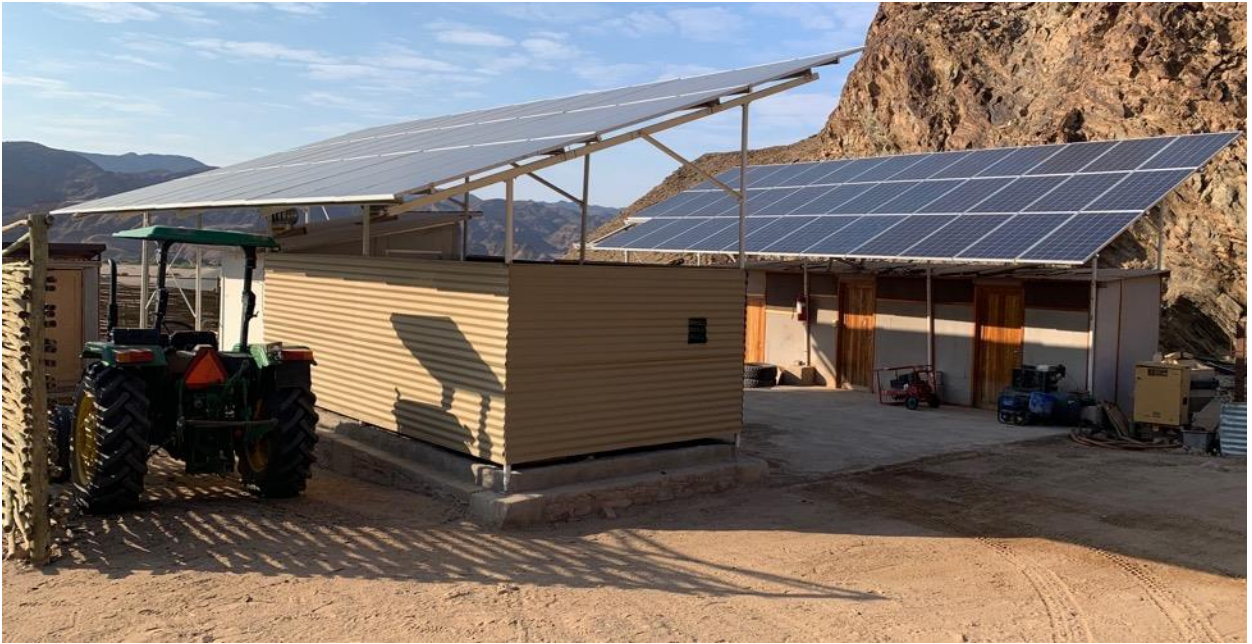
Figure 14. The PV array provides shade for maintenance store rooms.
