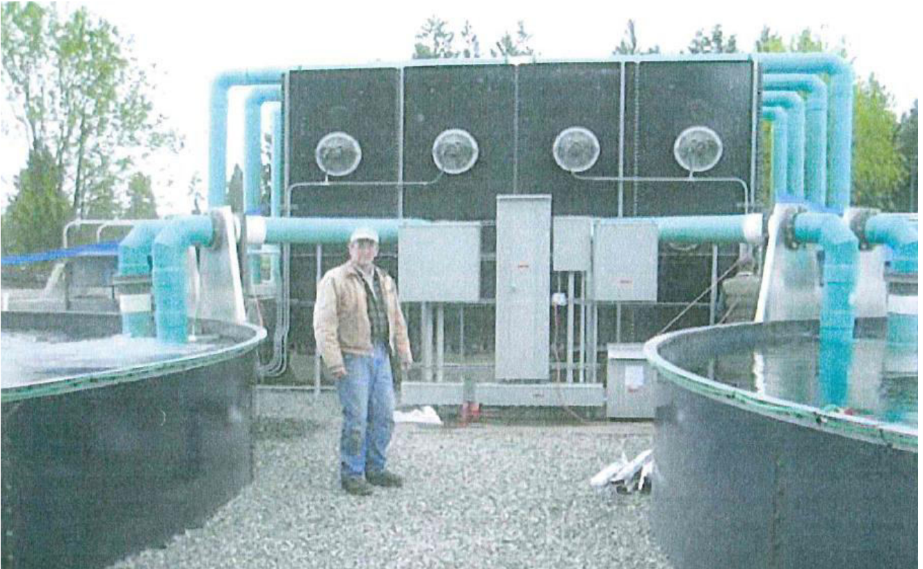
Plate 1.2: Example of typical HTE Beat Bio-filter and CO 2 stripper (Source: Atlantic Aquafarms (Pty) Ltd, 2015).
