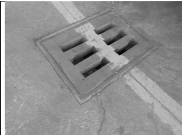
Image 1: Oil and water interceptor to collect wastewater and oils from the forecourt to the water and oil separator pits
