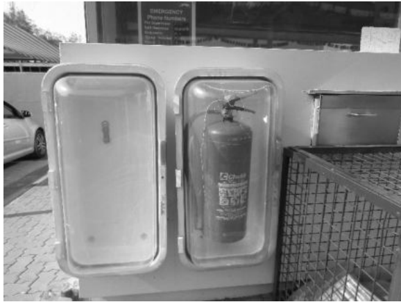
Image 1: one of the fire extinguishers on site.
