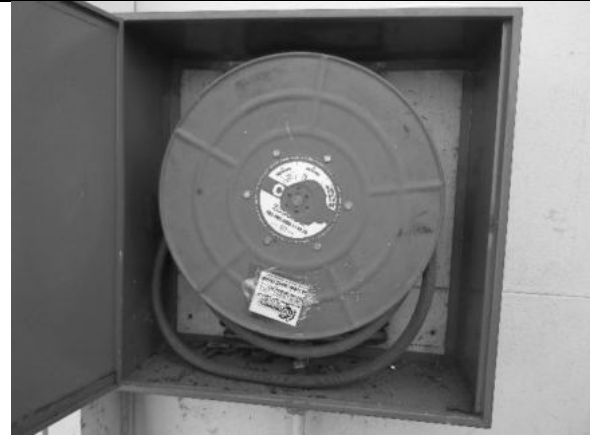
Image 4. Hose pipe on site
