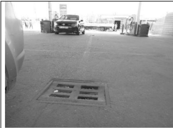
Image 1: Oil and water interceptor at filler points to collect wastewater and oils from the forecourt to the water and oil separator pits.
