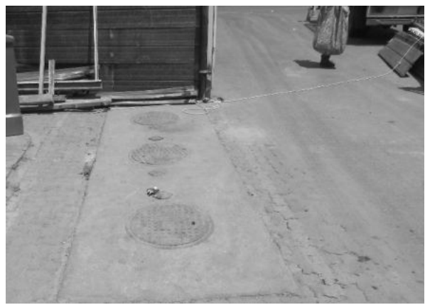
Image 2: Oil and water separator pits emptied regularly by certified contractors.
