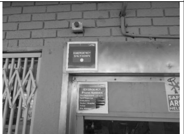
Image 4: emergency shutdown alarm.
