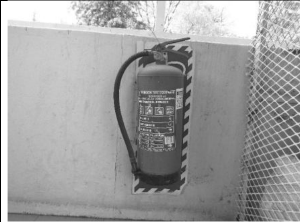
Image 1: One of the fire extinguishers on site.
