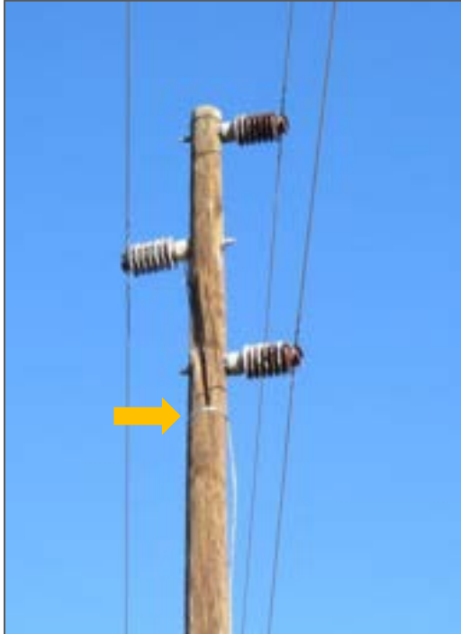
Figure 5-2: Example of "gapping" of a pole earth wire to provide an air space safety gap, in order to reduce the electrocution risk, The arrow indicates the upper limit of the earth wire.
