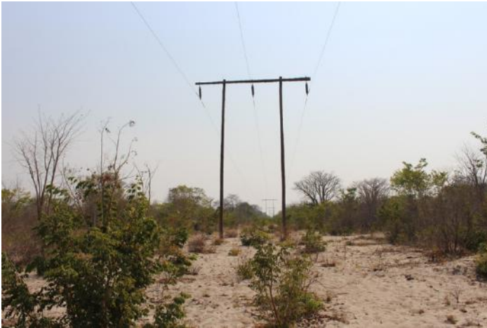
Figure 5: Powerline (Passing close to the project site)
