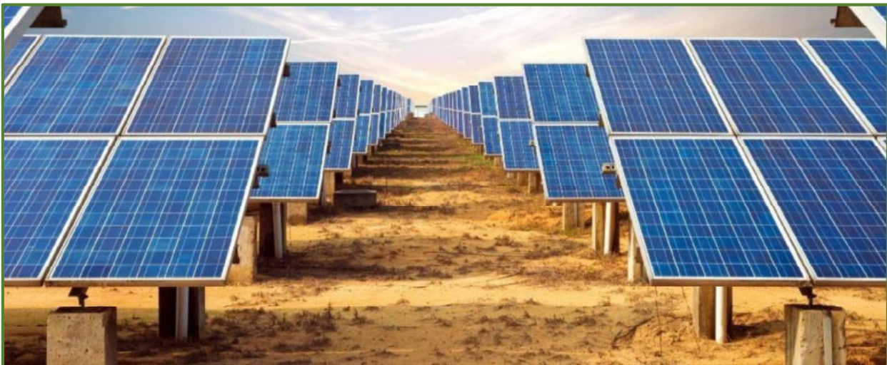
Figure 2: Illustrate the typical installation of solar panel filed, similar to which DanAon Energy envisage to install
