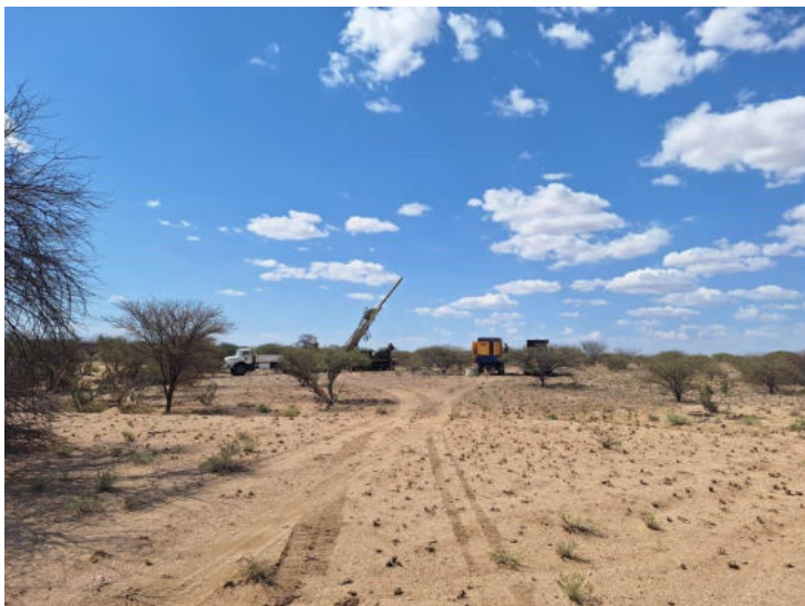
Figure 2 - Creation of new tracks to provide access to the various drilling sites.
