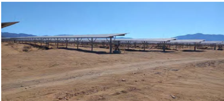
Photo 24 – View of installed solar panels with internal access road.
