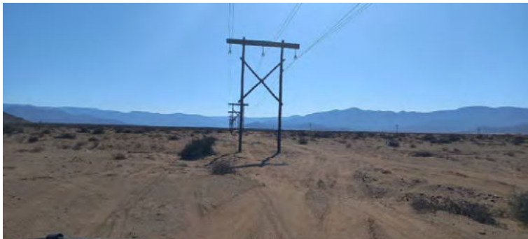
Photo 29 – View of OHTL extending from the PV plant to the main sub-station within Rosh Pinah. The OHTL will be monitored over the following months to determine any bird mortalities and applicable mitigations to be applied.
