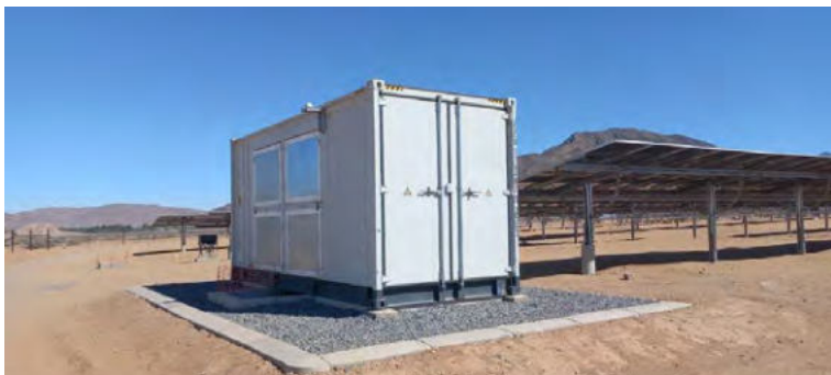
Photo 27 – View of containerised transformer.
