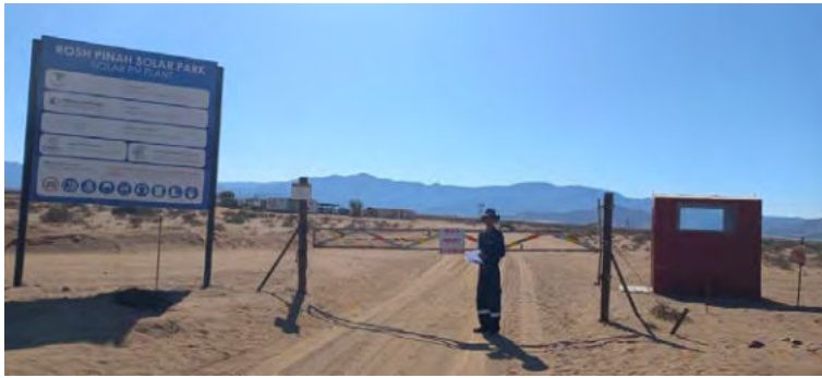
Photo 1 – View of access to Farm, Site Office & Construction Area with Project Information Board. Access is controlled and register is maintained.
