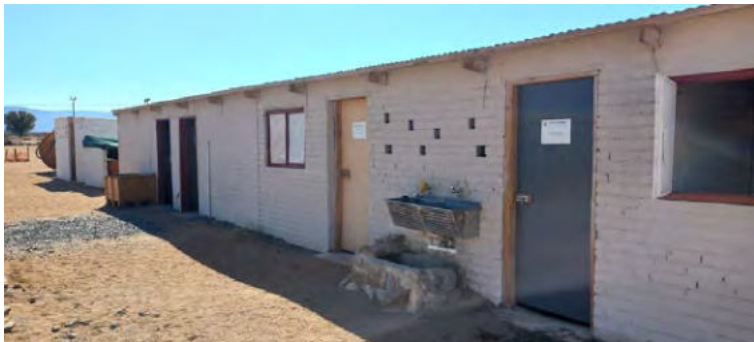
Photo 12 –View of site office's kitchen and ablution buildings at Contractor's Site Office. All kept in neat and tidy condition. Building provides for separate ablutions for men and woman, kitchen and locker rooms.
