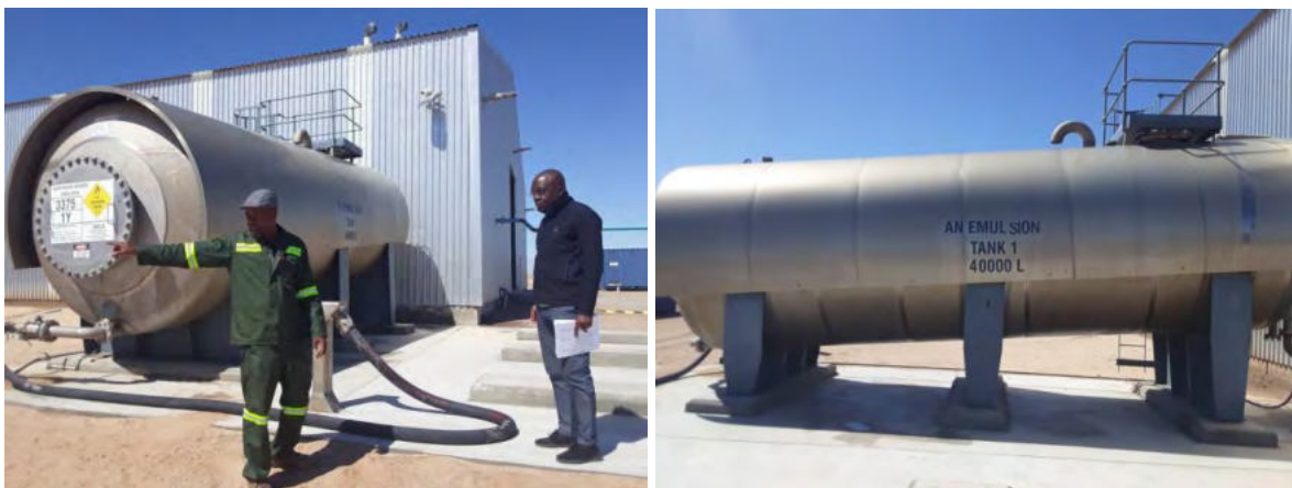
Figure 2: Ammonium Nitrate Emulsion Storage Tank
