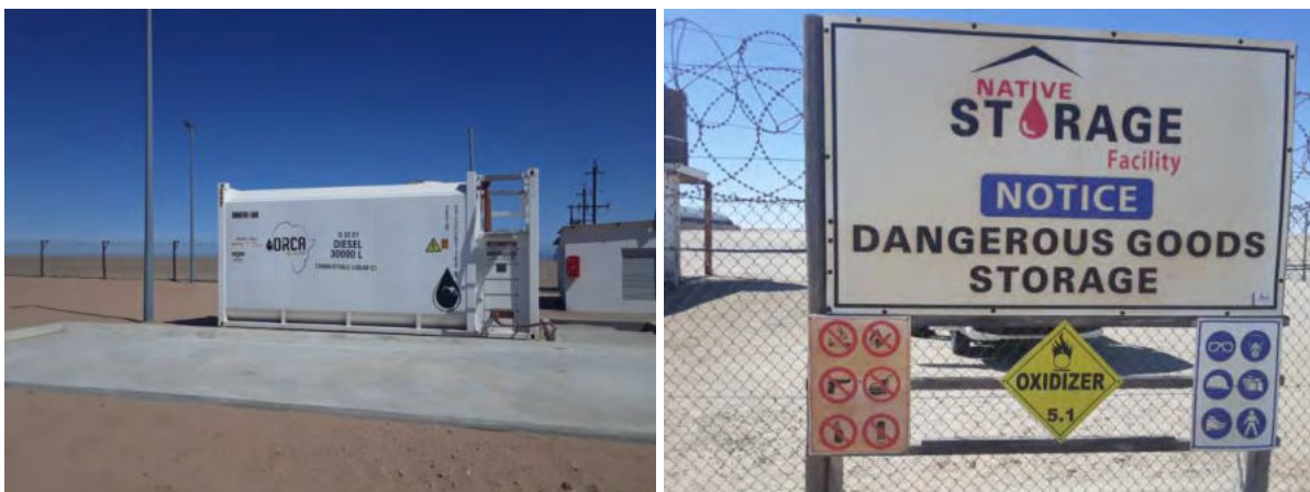
Figure 3: Self-bunded Diesel Fuel Tank and Signage
