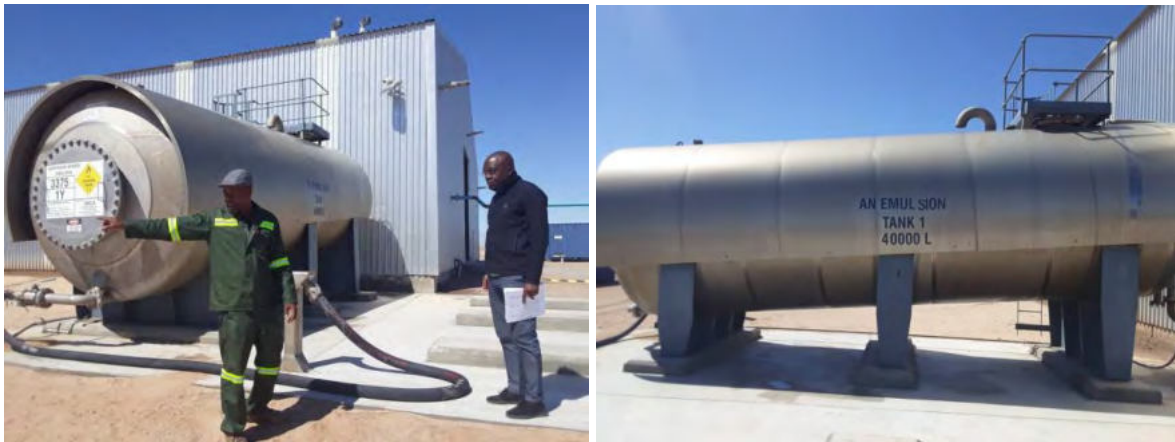
Figure 2: Ammonium Nitrate Emulsion Storage Tank
