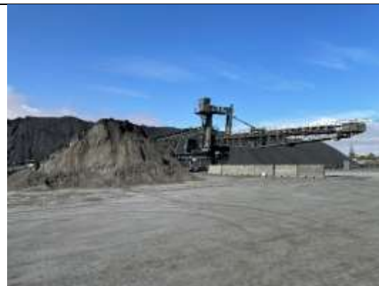
Photo 4-10 Mobile conveyer unit inside storage yard
