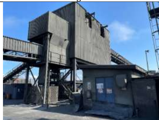
Photo 4-8 Conveyer lines splitting at the entrance to the storage area
