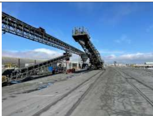
Photo 4-5 Conveyer line at the dock. Note it is not closed off on the side
