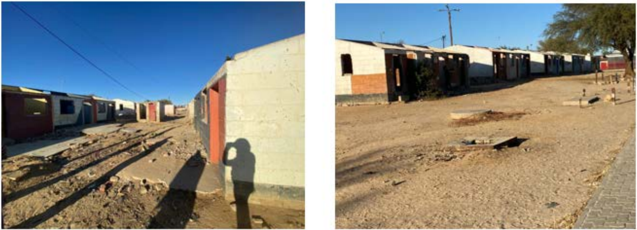
Figure 4: Dilapidated State of the neighboring dwellings
