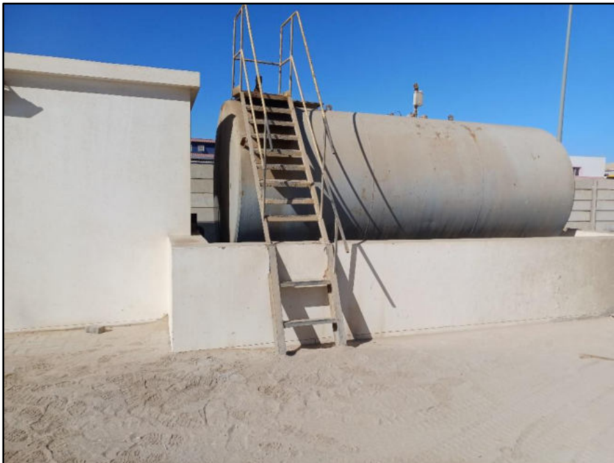
Figure 6: Bunded steel tank
