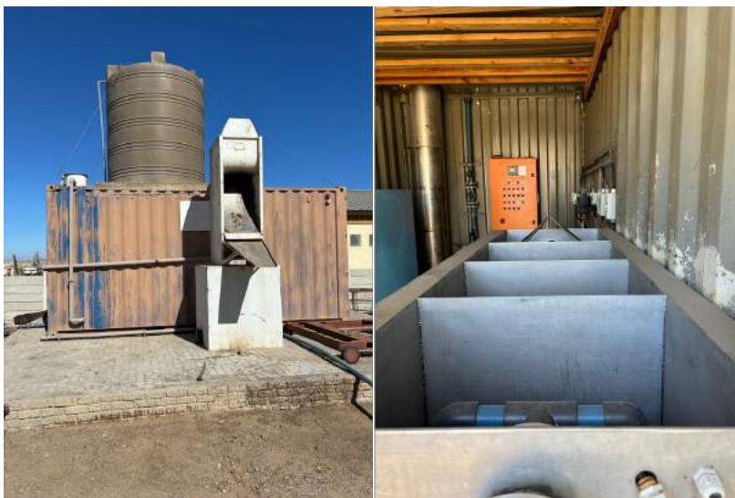
Figure 2: Aqua Treatment Plant
