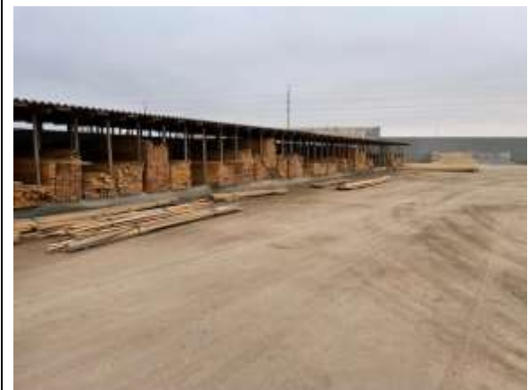
Photo 4-2 A view of the northern boundary and roof that is to be demolished
