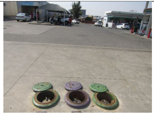
Image 2: A concrete slab around the tanks area and dispensing points for surface spills containment
