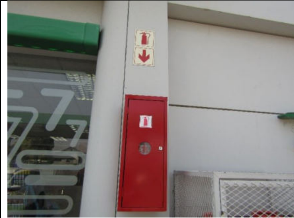
Image 1: one of the fire extinguishers on site.
