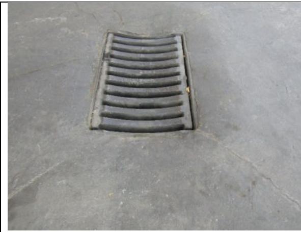
Image 1: Oil and water interceptor at fuel dispensing points to collect wastewater and oils from the forecourt to the water and oil separator pits
