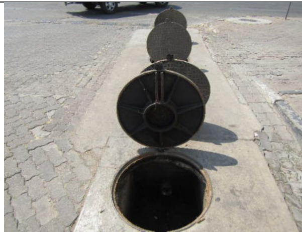
Image 2: Oil and water separator pits emptied regularly by certified contractors.
