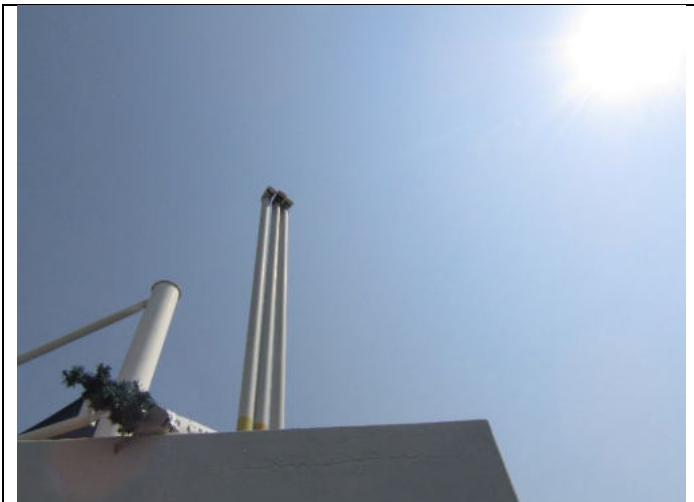
Image 1: Vent pipes have been installed on site (3m) to release vapors above the immediate atmosphere to enhance pollution attenuation.
