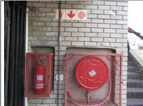
Image 1: one the fire extinguishers and hose pipes on site.
