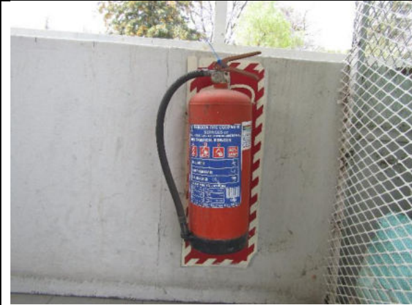
Image 1: One of the fire extinguishers on site.
