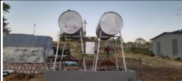
Photo 4-21 Fuel storage tanks
