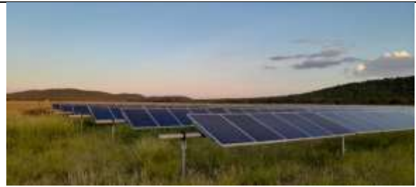
Photo 4-20 Photovoltaic solar system
