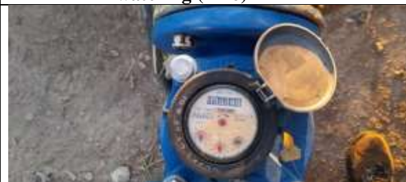
Photo 4-36 Water meter installed at irrigation borehole (EB1 / WW40210)
