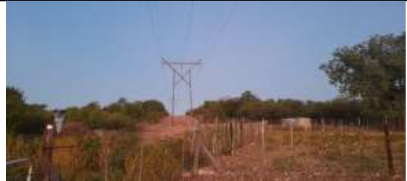
Photo 4-22 66 kV power line on site
